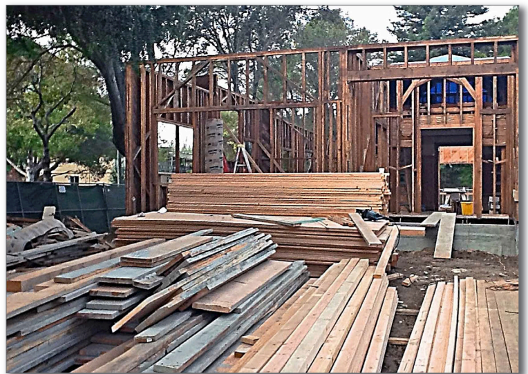
The original first floor framing of this deconstructed house remains in place on a new foundation, January 2014. Recycled lumber on the left is from a different house. Photo: Naphtali H. Knox, FAICP.
