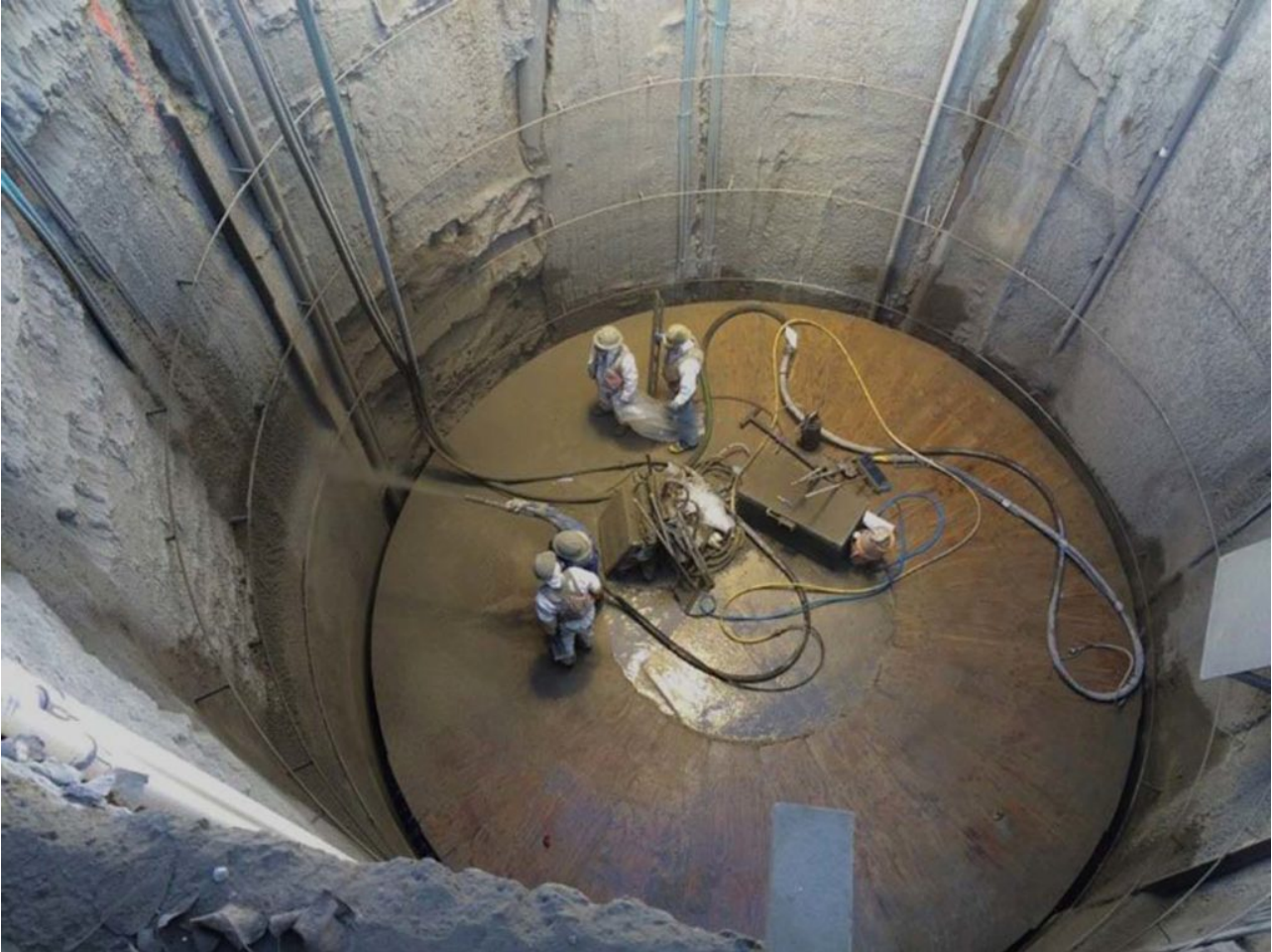
One of three vertical shafts being excavated for the project. The tunnel-boring machine will be lowered into the first shaft and will begin excavating the tunnel horizontally. Photo: Silicon Valley Clean Water.
